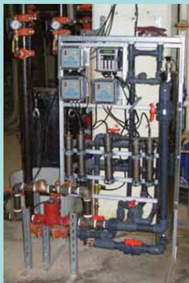
A typical eH 2 O non chemical water treatment system on a 1000 ton HVAC cooling tower.
