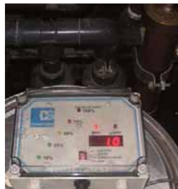
Above Rates in the 1 Mil Per Year range is typical with eH 2 O water treatment. This is an excellent corrosion rate for mild steel.
