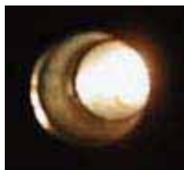
Above A clean tube bundle with inspection. Perfectly clean tube bundles are what you see with eH 2 O tube bundle inspections. Machine temperatures also validate the performance of the system.
